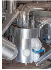
Streekpellets white pellet plant, The Netherlands, 2018 - 2020 Capacity: 10 kton/a
