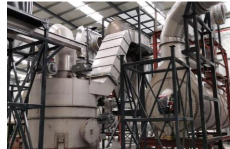
Futerra - 6 lines torrefaction plant Portugal, 2019 - 2021 Capacity: 120 kton /a
