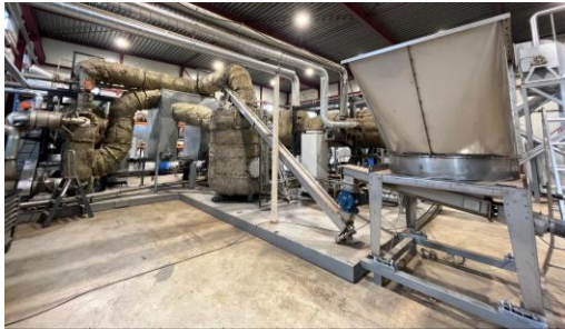
Demonstration plant in Ruurlo, The Netherlands, 2017 - Today Capacity: 0,25 tons per hour
